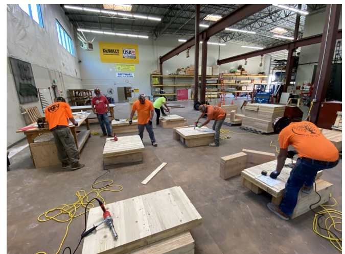
Above: Carpenters use shop drawings and standard tools to prepare and assemble the WoodWorks-provided mass timber components at the 8/14/2020 installation training workshop in Kent, WA.
